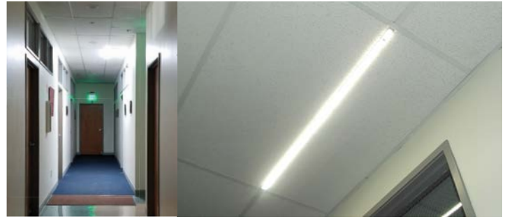
Power outage- emergency LEDs activated
