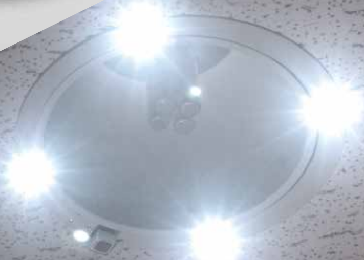
HOTSPOT1 IN OPERATION DURING POWER OUTAGE
